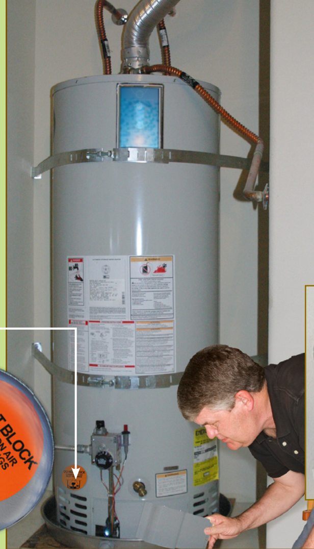
FVIR Water Heater
