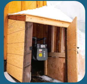
METER WITH SNOW SHELTER
